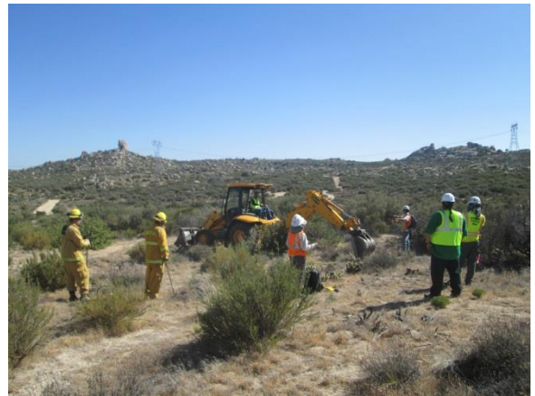
Photo 4: ECMs observed fire patrols from San Diego Rural Fire District monitoring backhoe activity at each geotechnical location. Areas of activity were pre-wetted in accordance with the conditions the NTP and fire patrols were observed conducting fire watch one hour following geotechnical activity areas.
