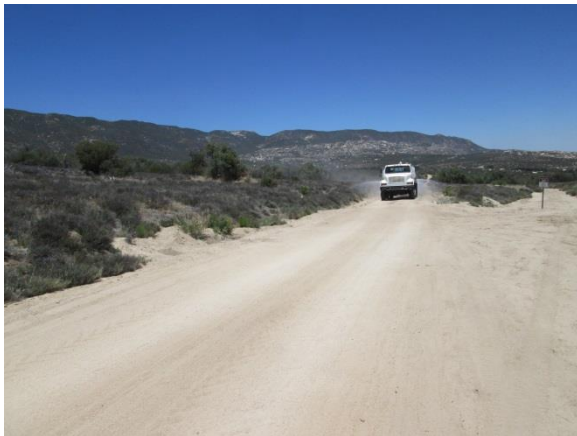
Photo 3: A water truck applies water to McCain Valley Road in order to suppress any potential fugitive dust resulting from geotechnical activity traffic in accordance with the conditions in NTP-1.
