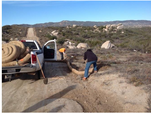
Photo 2: Crews installing additional straw wattles along McCain Valley Road in accordance with the SWPPP and MM HYD-1.
