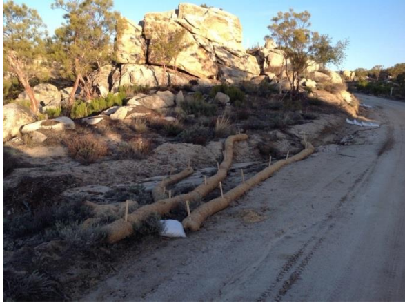
Photo 1: Previously installed erosion control devices along McCain Valley Road reinforced with an additional sand bag and straw wattle following the site-wide SWPPP inspection in accordance with the SWPPP and MM HYD-1.
