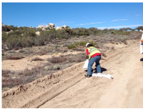
Photo 4: Crews installing additional sand bags at areas subject to overland flow during rain events along McCain Valley Road in accordance with the SWPPP and MM HYD-1.
