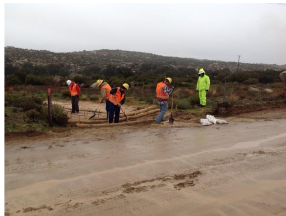
Photo 4: Crews installing additional straw wattles and maintaining existing erosion and sediment control devices along McCain Valley Road in accordance with the SWPPP and MM HYD-1. Cultural monitors were present to observe ground disturbance associated with the installation and maintenance of sediment control devices in accordance with MM CUL-1D.
