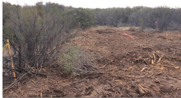
Photo 2: On 1.11.17, approximately 230 square feet of vegetation was mulched outside of the limits of disturbance. This event is being classified as a "Non Compliance" in accordance with Section 5.2 of the ECCMP.
