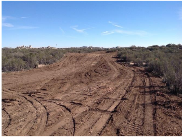
Photo 1: On 1.18.17, approximately 11,700 square feet of vegetation was mulched outside of the currently approved limits of disturbance. BLM issued a “Non Compliance” in accordance with Section 5.2 of the ECCMP.
