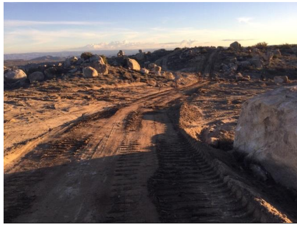
Photo 2: On 1.16.17, a BLM third party cultural monitor observed a blade operating in a previously disturbed area along the G string access road between structures G7 and G6 without a cultural monitor present. BLM issued a “Non Compliance” in accordance with Section 5.2 of the ECCMP.
