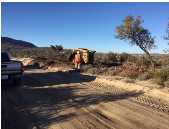
Photo 3: Cultural monitors were observed monitoring vegetation removal and grading activities along McCain Valley Road in accordance with MM CUL-1D.
