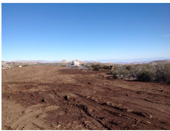
Photo 4: Water trucks were observed working alongside grubbing machines in accordance with the approved Fire Prevention/Protection Plan (MMs FF-1 and BIO-1F).
