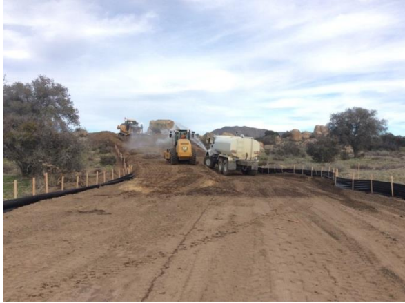
Photo 1: Clearing and grading activities observed within the staked limits of disturbance in accordance with MM BIO-1A. Water trucks in use for dust control in accordance with MM-AQ-1.
