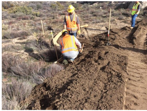
Photo 4: Crews installing additional straw wattles along McCain Valley Road in accordance with the SWPPP and MM HYD-1.
