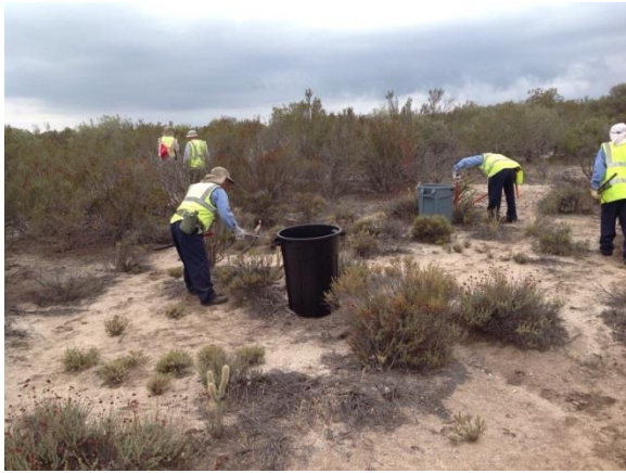
Photo 1: Crews using hand tools to salvage cacti on the access road from McCain Valley Road to turbine G5 in accordance with LNTP-2 authorized activities and the Habitat Restoration Plan (MM-BIO-1D).
