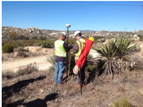
Photo 3: Survey crews staking grading limits along McCain Valley Road in accordance with MM BIO-1A.
