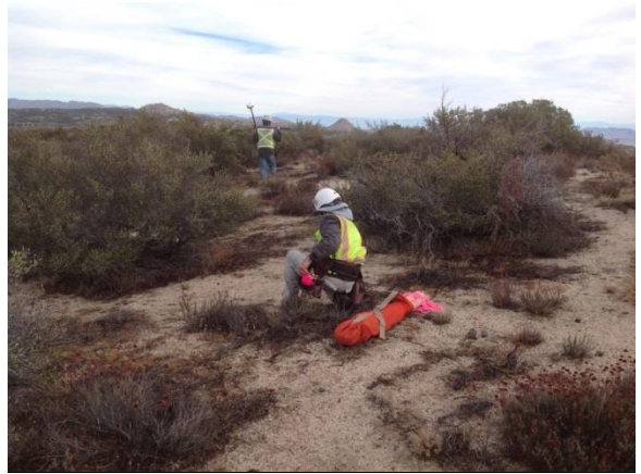
Photo 2: Westwood survey crews staked the center line of the road on the C String ensuring the limits of the work area are delineated in the field according to the development plans (MM BIO-1A).
