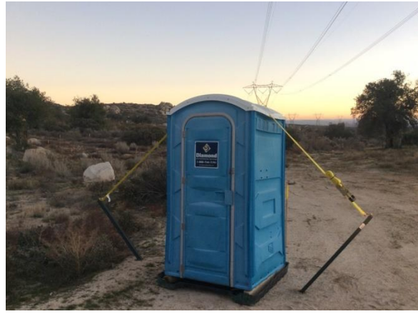
Photo 2: Portable restroom facilities are staked to the ground surface with containment in place to prevent the potential for leaks or spills in accordance with ROW Grant Stipulation 78 and the Hazardous Materials Management Plan.
