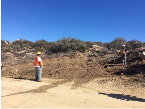
Photo 1: Archaeological and Native American monitors present during clearing and grading activities for the installation of water tanks along McCain Valley Road (MM-CUL-1d).
