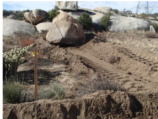
Photo 4: A boulder was pushed approximately 15 feet outside of the limits of disturbance. This event is being classified as a "Problem Area" in accordance with 5.2 of the ECCMP.
