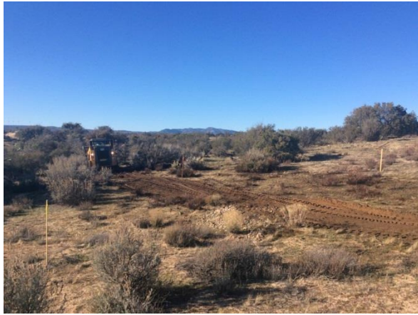
Photo 1: Clearing and grading activities observed within the staked limits of disturbance in accordance with MM BIO-1A.
