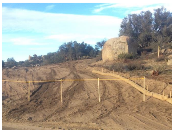
Photo 4: Temporary fencing installed to discourage unauthorized use of construction roads during the holiday break.
