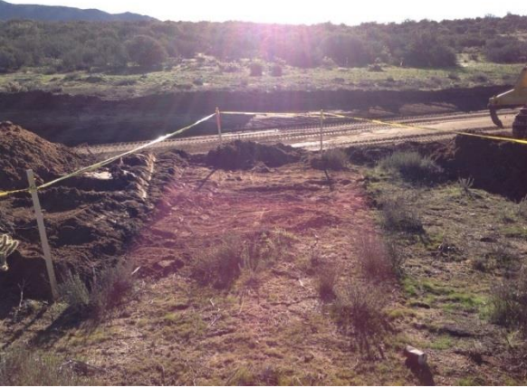
Photo 1: On February 9, 2017, ECMs observed a noncompliance event where an equipment operator caused disturbance beyond the limits of disturbance by first pushing soil outside the limit and then back-dragging the soil back into the limits of disturbance.
