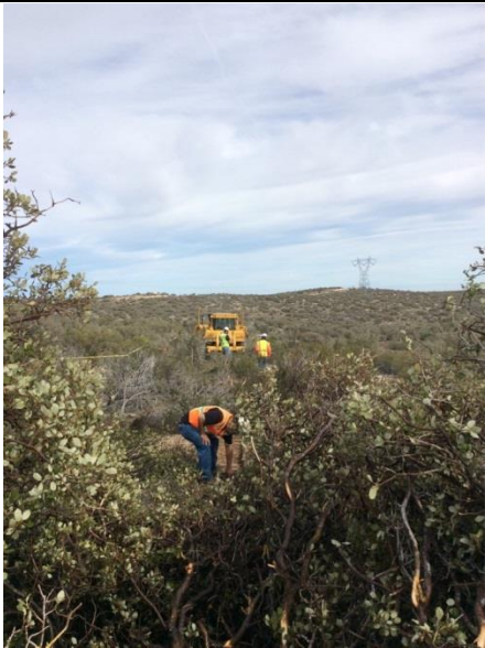
Photo 3: Resource monitors and equipment operators cut pre-grubbing lines in thick vegetation along the yellow tape disturbance limits with monitors acting as spotters ahead of the equipment in accordance with the February 1, 2017 NTP.
