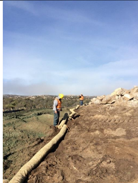
Photo 4: Crews observed installing erosion and sediment control devices around salvaged topsoil stockpiles in accordance with the Habitat Restoration Plan and Section 7.8 of the SWPPP.
