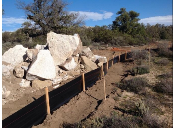
Photo 2: During this reporting period, crews repaired a damaged silt fence on the McCain Valley cutoff road per direction provided by the QSP and ECMs in accordance with the SWPPP.
