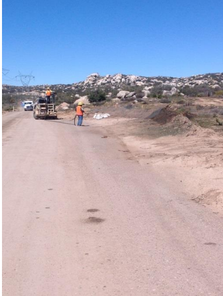
Photo 3: ECMs observed construction crews hydromulching topsoil salvage windrows along McCain Valley Road in accordance with the SWPPP.
