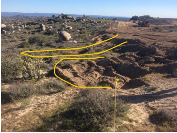
Photo 1: On March 13, 2017, disturbance beyond the staked limits of disturbance occurred when a piece of construction equipment hit a subsurface rock and lost control. The area of disturbance was inspected and it was determined that no damage to sensitive environmental resources occurred.
