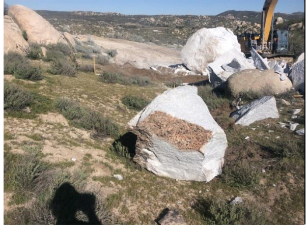
Photo 2: During blasting activities on March 16, 2017, rock debris fell approximately 10 feet outside the staked disturbance limits. The pieces of rock were left in place to avoid creating additional unauthorized disturbance.
