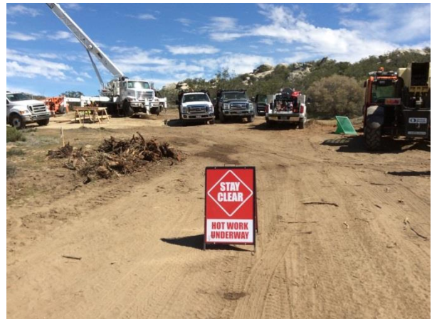
Photo 4: Required equipment and warning signs were present at the Transmission Line Pole 4 during hot work activities in accordance with the issued hot work permit and the Fire Prevention/Protection Plan (MM FF-1).
