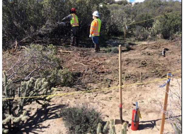
Photo 2: Fire prevention equipment was staged within 30 feet of chainsaw work along the collection line in accordance with the Fire Prevention/Protection Plan (MM FF-1).
