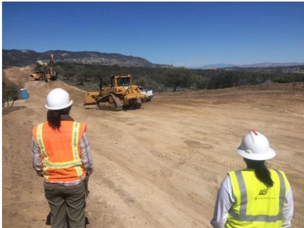
Photo 3: Archaeological and Native American monitors were present during grading activities along McCain Valley Road in accordance with MM CUL-1D.
