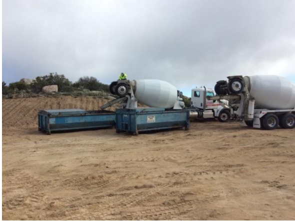
Photo 1: Concrete washout containers were used during foundation pouring activities to ensure contaminated discharge was contained in accordance with MM BIO-5.
