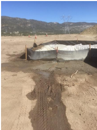
Photo 3: ECMs observed excess concrete/water mixture outside of the silt fencing in multiple locations. The construction contractor was notified to install gravel aprons in accordance with the Grading Plans (please see Photo 4) and to not fill washout basins beyond capacity.
