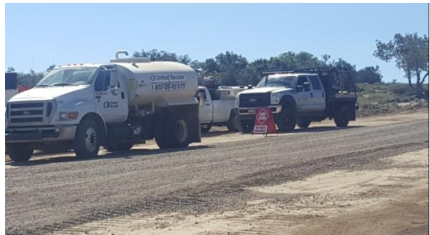
Photo 2: A water truck, fire safety coordinator, and identification signage are located where hot work was occurring in accordance with MM FF-1.
