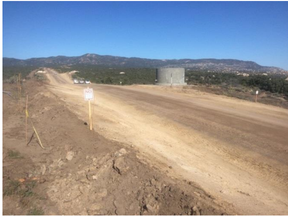
Photo 1: Nesting black throated sparrow ESA at tank 3, within which a Blattner crew was accidentally given permission to work by the ICF designated biologist when signing MSOS documents for the activity. Following identification of the issue, a biological monitor was assigned to the activity in accordance with MM BIO-7j and no impacts to the active nest were observed.
