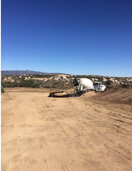
Photo 3: ECMs observed the concrete washout at turbine pad G15 without a rock apron as required by design detail WM-8 included in the grading plans. ECMs notified Tule Wind, LLC of the problem area. A rock apron is anticipated to be installed in accordance with the grading plans.
