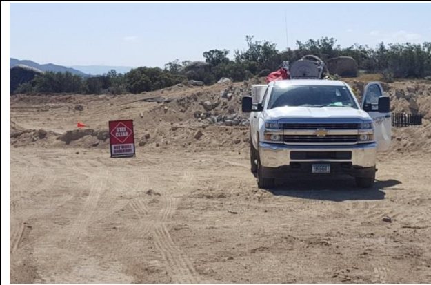
Photo 1: Fire safety coordinator and required signs were present during Hot Work at turbine pad G12 in accordance with the issued Hot Work Permit and MM FF-1.
