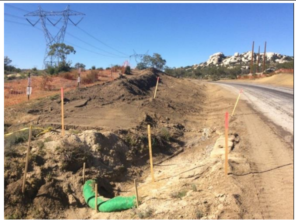
Photo 2: Erosion and sediment control ditches and straw wattles were installed along McCain Valley Road in accordance with the SWPPP.
