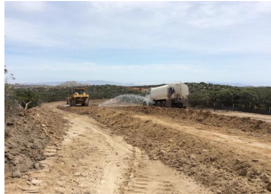
Photo 4: ECMs observed road grading on the access road between pad sites C2 and C5 with an accompanying water truck in order to minimize fugitive dust as per MM AQ-1. Yellow tape is shown marking limits of disturbance in accordance with the February 2, 2017 NTP.
