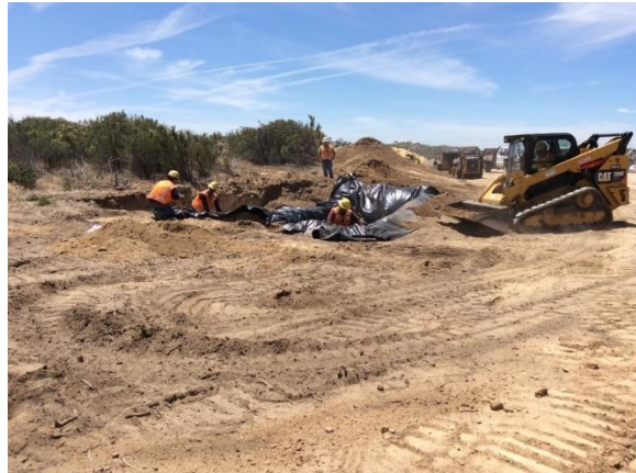
Photo 4: The new concrete washout pits at Yard 6 were double-lined with thick poly sheeting to prevent soil contamination in accordance with MM HYD-1 and the project SWPPP.
