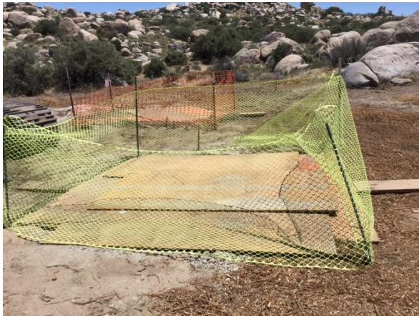
Photo 3: Excavations are covered to prevent wildlife from becoming entrapped in accordance with MM BIO-7A.
