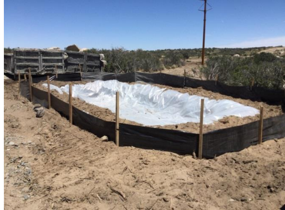
Photo 2: The silt fencing surrounding a concrete washout basin is maintained in good condition. A rock apron is anticipated to be installed at the washout basin in accordance with figure WM-8 of the grading plans.
