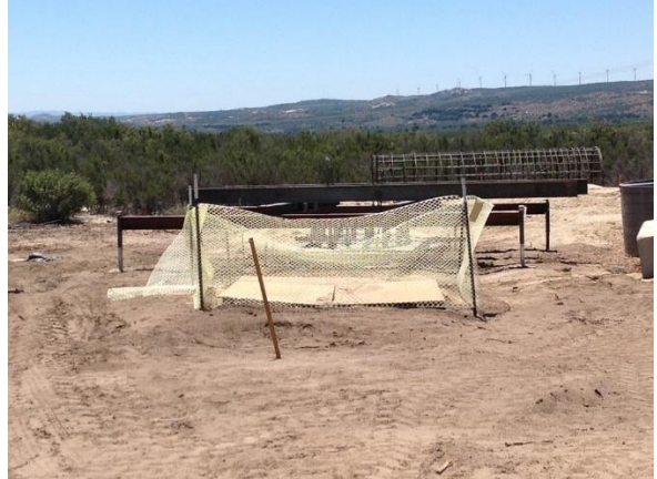
Photo 4: ECMs observed inactive excavations covered to prevent entrapment of wildlife in accordance with MM BIO-7A.
