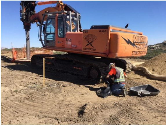
Photo 1: ECMs observed a construction crewmember cleaning up stained soil at collector pole site 27 in accordance with MM HAZ-1A.
