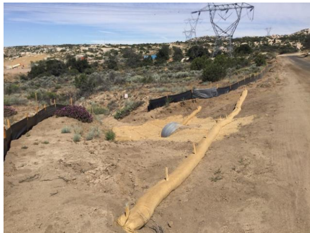
Photo 3: Erosion blankets and biodegradable straw wattles are installed along culverts in accordance with MM-HYD-4 and site specific SWPPP.
