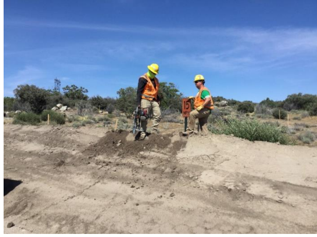
Photo 2: A construction crew is observed adding a speed limit sign along McCain Valley road in accordance with MM-TRA-1.
