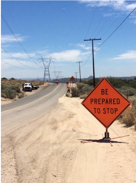
Photo 1: ECMs observed traffic flaggers present and signage posted at the entrance of McCain Valley Road in accordance with MM-TRA-1.
