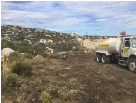
Photo 3: ECMs observed a water truck present during vegetation removal and grubbing at collector pole #31 in accordance with MM-AQ-1. Native American and archaeological monitors present but not pictured.
