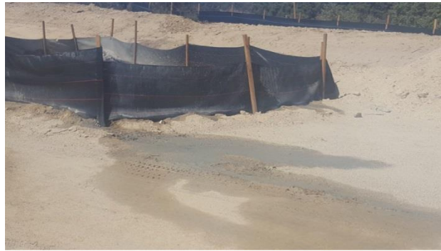
Photo 1: On August 4, 2017, ECMs recorded concrete washout that had flowed outside the established washout containment and silt fence along C line. The designated biologist was notified.
