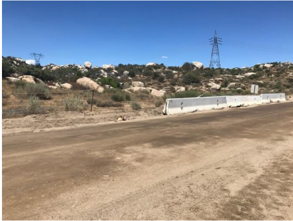
Photo 3: ECMs observed K-rails placed along McCain Valley Road to protect an established ESA during component delivery and additional road work in accordance with the approved Variance Request 010.
