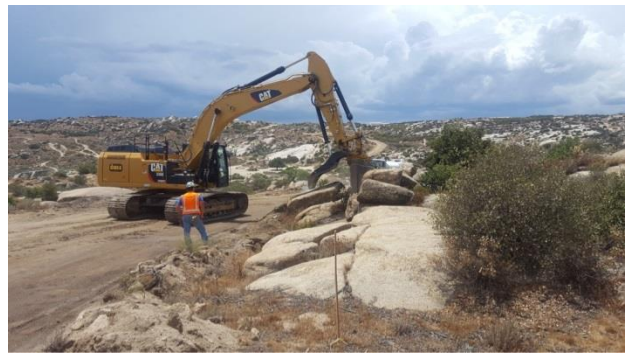
Photo 4: During this reporting period, ECMs and applicable monitors were present to perform preconstruction inspections and required monitoring of the rock relocation outside of work limits north of J line in accordance with the approved Variance Request 006.
