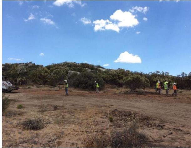
Photo 1: ECMs observed biological and cultural monitors conducting sweeps ahead of a skid steer during electrical line pulling for transmission pole 4, in accordance with MM-CUL-1d.
