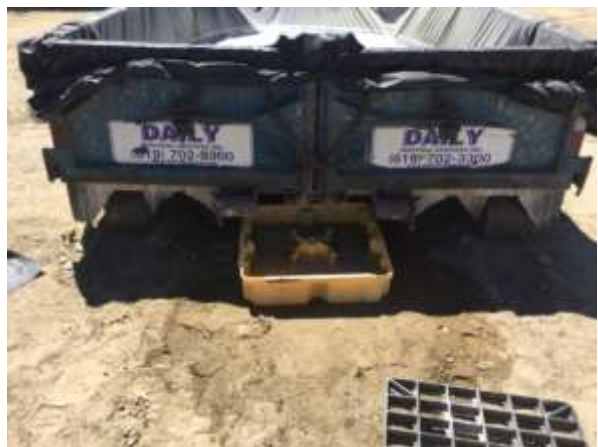
Photo 4: During this reporting period, ECMs notified the designated biologist that the concrete washout containment at turbine pad G4 was leaking. Following notification, a containment bin was placed under the leak, but the stained soil remained onsite.
