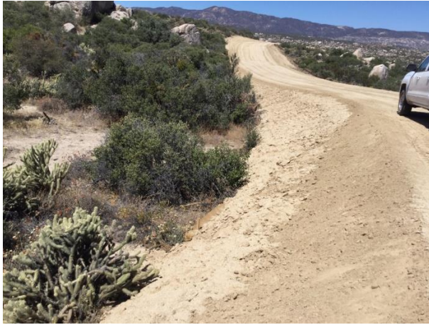
Photo 1: ECMs observed straw wattles buried beneath soil at the entrance to turbine site D-2. The designated biologist was notified of the issue and ECMs will continue to monitor this issue.
