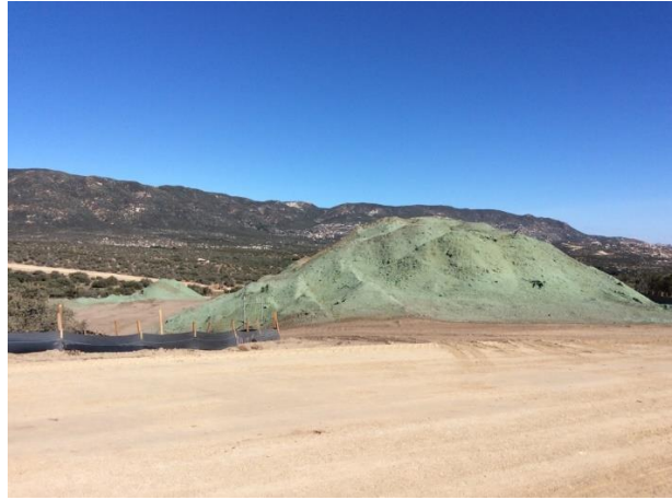
Photo 2: ECMs observed top soil piles at laydown yard #2 stabilized with a soil binder to help minimize top soil erosion in accordance with section 7.3 of the site specific SWPPP.
