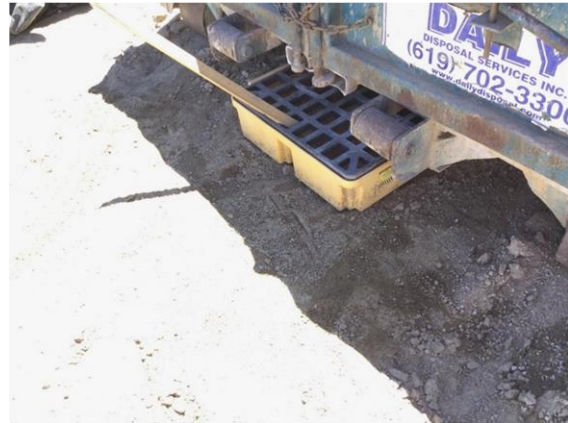
Photo 4: ECMs observed containment bins beneath roll off dumpsters being used as temporary washout basins to prevent washout from leaking onto the ground surface.
