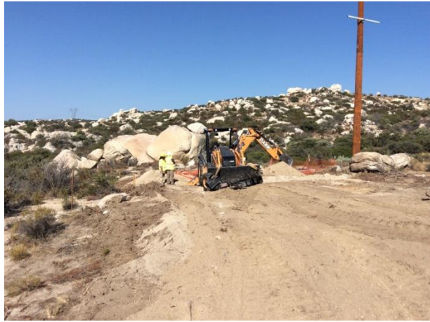
Photo 1: Full-time archaeological and Native American monitors were present during trenching activities at overhead collection pole 31 in accordance with MM CUL-1d.
