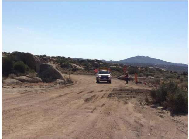
Photo 2: Flaggers were present during turbine component hauling on McCain Valley Road in accordance with MM TRA-1.
