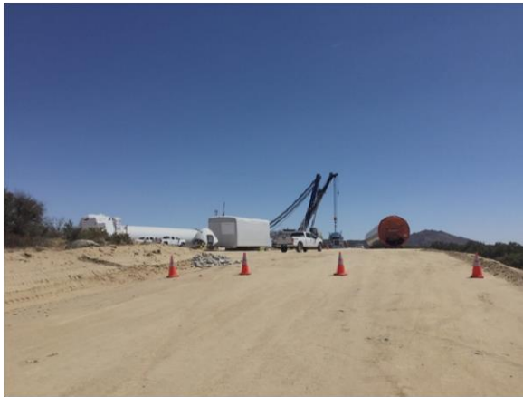
Photo 3: ECMs observe turbine assembly from a safe distance. Construction crews use cones to implement safety stand-off distances and safe working practices detailed in MM HAZ-1b and MM TRA-1.
