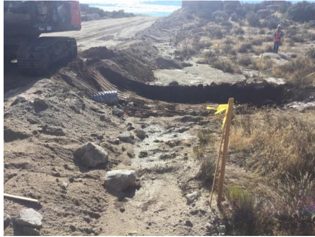
Photo 1: ECMs observed construction crews excavating adjacent to culverts for the installation of rip rap in accordance with the site specific SWPPP and MM HYD-1.
