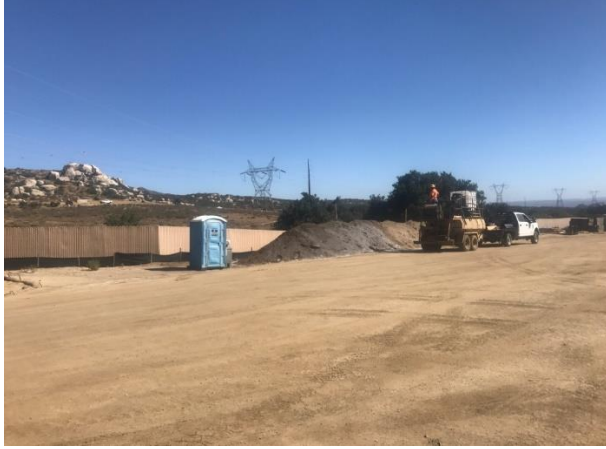
Photo 1: ECMs observed construction crews applying soil binders to soil piles in the 80-acre laydown yard to prevent wind erosion, in accordance with the site specific SWPPP and MM HYD-1.
