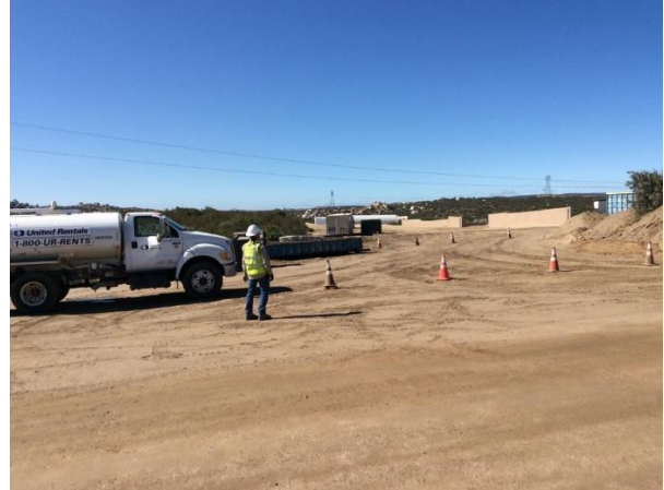
Photo 2: ECMs observe a construction crewmember at a temporary road closure to allow overhead collector lines to be safely pulled over the right of way in accordance with MM TRA-1.
