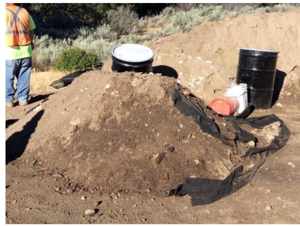
Photo 4: ECMs observed a stained soil pile from an equipment leak. Soil was held on a fabric mat to keep contaminants from contacting the ground. The pile was later cleaned and removed in accordance with MM HAZ-1a.
