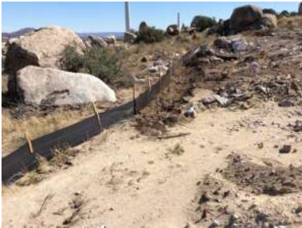
Photo 3: ECMs observed a repaired silt fence from a previous reporting period, in accordance with the project SWPPP and MM HYD-1.
