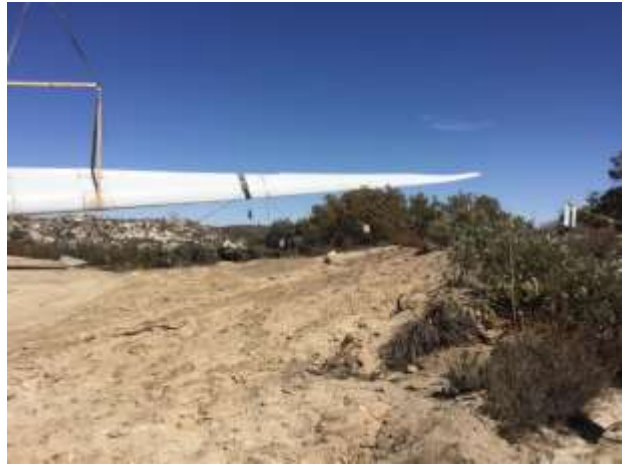
Photo 2: ECMs observed turbine blade assembly at pad G-14. Blades extended approximately 65 feet outside the limits of disturbance. Before installation continued, the area was cleared per the protocols of Variance Request 006. The area was swept by biological and cultural monitors along with third party ECMs to ensure no biological or cultural resources were affected.
