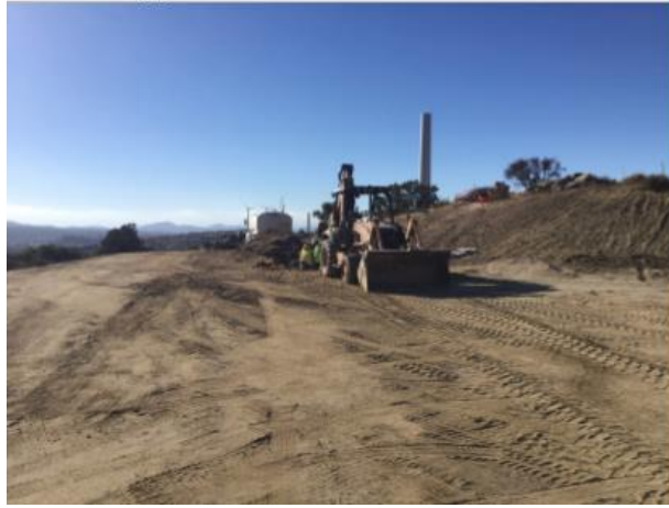
Photo 1: ECMs observed trench backfill at turbine pad G-7. A water truck was present during activity to minimize dust in accordance with MM AQ-1 and the dust control plan.
