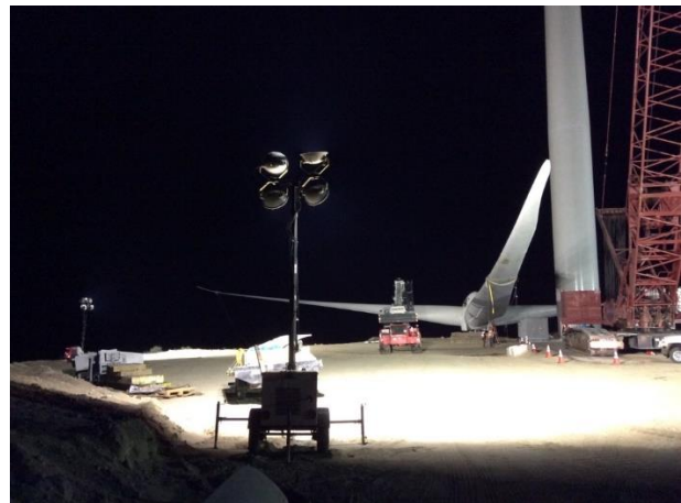
Photo 4: ECMs observed light plants appropriately positioned down and in towards construction activities, to minimize lighting in adjacent native habitat and illumination into the nighttime sky, in accordance with MM BIO-7C, APM BIO-15 and MM VIS-3B.
