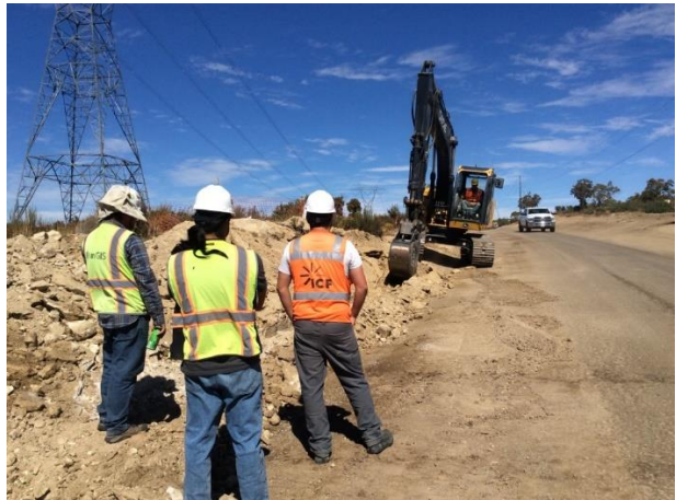
Photo 3: Archaeological, Native American, and Biological monitors observe construction crews cutting a drainage ditch along McCain Valley Road, in accordance with MM CUL-1D, MM BIO-1C, and the approved Tribal Participation Plan.
