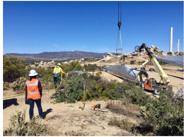
Photo 2: ECMs observed fire crews presoaking vegetation prior to removal at turbine pad G-12 to accommodate turbine blade installation in accordance with MM FF-1. ASM cultural resource monitors, ICF biological monitors, and third party ECMs implemented the requirements of Variance Request 006 after discussing vegetation removal with a Habitat Restoration Specialist.
