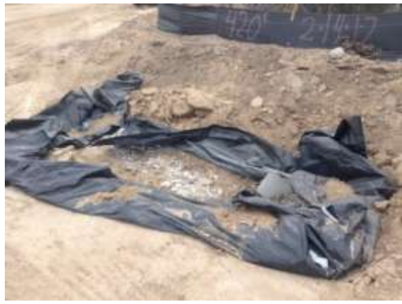
Photo 2: ECMs observed a wash out basin near turbine pad F-2 in poor condition. ECMs coordinated with the designated biologist to repair the wash out basin, in accordance with the project site specific SWPPP.
