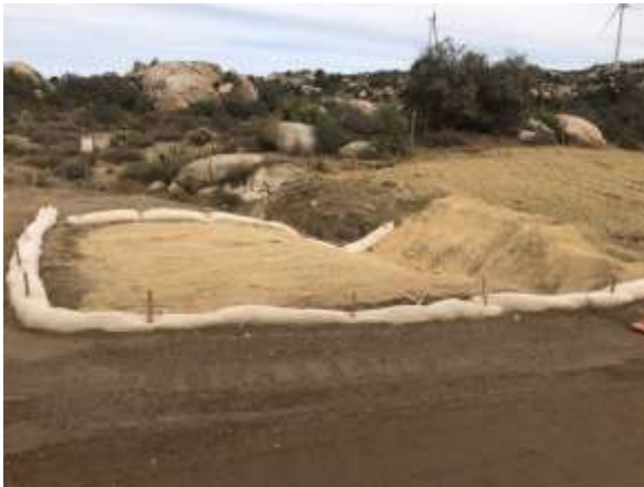
Photo 3: Installation of straw wattles and fiber blankets continued along McCain Valley Road, in accordance with the project site specific SWPPP and MM HYD-1.
