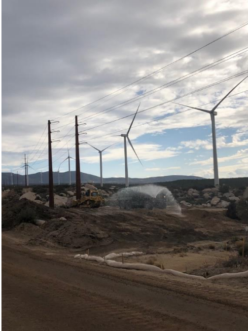
Photo 1: An ECM observed a water truck applying water during earthwork activities to control and minimize dust in accordance with MM AQ-1 and the Dust Control Plan.
