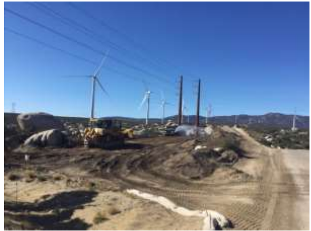
Photo 2: Reclamation/re-contouring activities occurred at overhead collector pole site 23. A water tender applied water in an effort to minimize dust in accordance with MM AQ-1.
