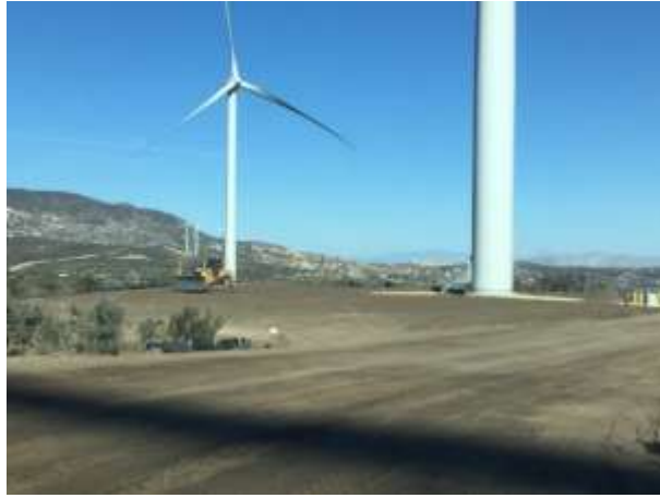
Photo 1: A bulldozer is observed spreading topsoil at turbine pad C-2 in accordance with Section 5.2 of the Habitat Restoration Plan.
