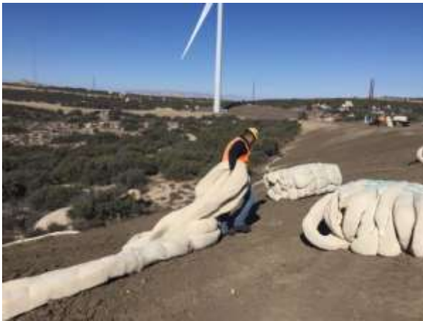
Photo 3: A construction worker is observed installing straw wattles along the slope at turbine pad E-10, in accordance with site specific SWPPP.
