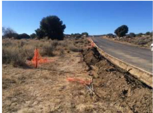
Photo 4: Looking west along Rough Acres Ranch Road where ESA fencing was removed and trenching occurred without an archaeologist or Native American monitor present. This incident was documented as a serious violation by the BLM.
