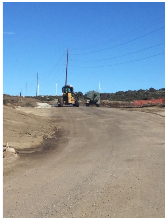
Photo 4: ECMs observed equipment blading the southern sections of McCain Valley Road. This activity was spot checked by archaeological and Native American monitors in compliance with MM CUL-1d.
