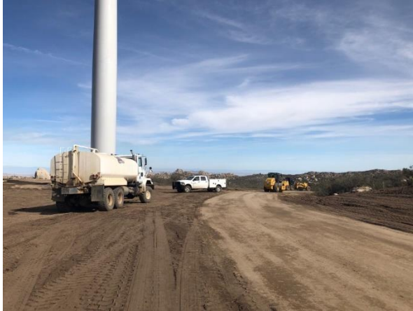
Photo 1: A water tender is observed applying water along a blade and roller near turbine pad D-2 in an effort to minimize dust in accordance with the Dust Control Plan and MM AQ-1.
