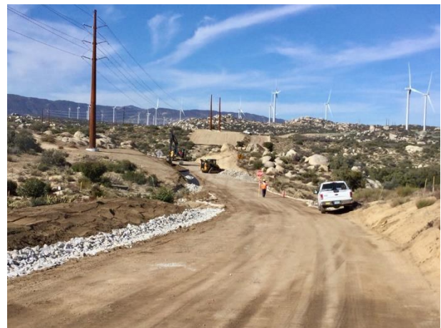
Photo 4: Construction crewmembers are observed installing a rock lined ditch along McCain Valley Road with traffic control being implemented in accordance with MM TRA-1.
