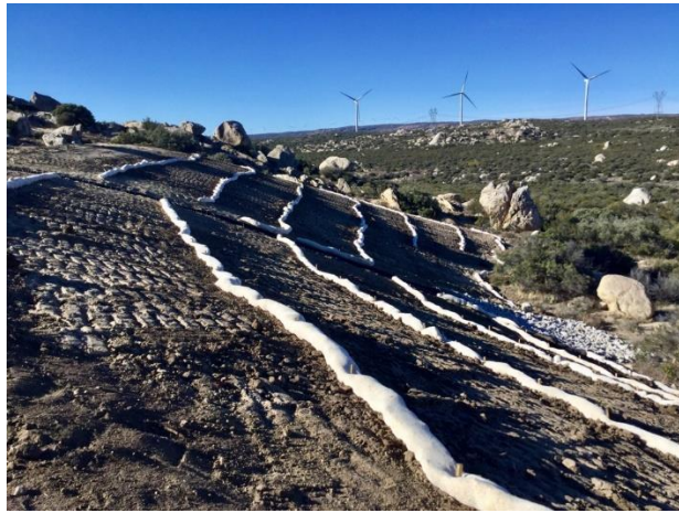
Photo 1: Straw wattles and other BMPs at turbine site E-10 have been reinforced, in accordance with site specific SWPPP.
