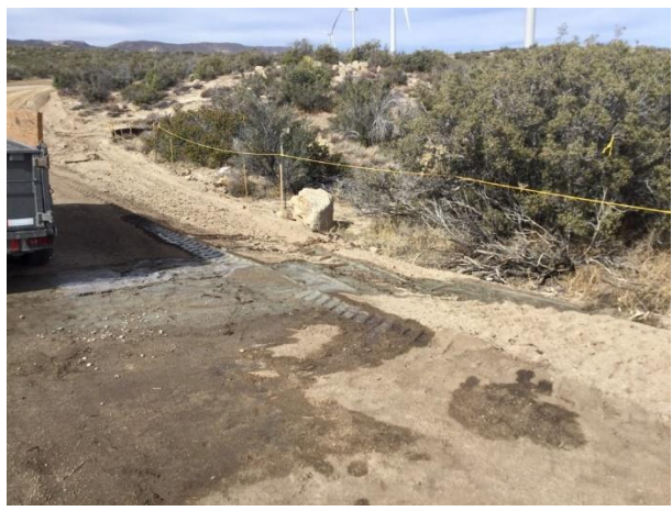
Photo 2: ECMs observed a concrete washout leaking from a temporary roll-off bin at turbine pad C-8. Construction personnel were immediately notified and the spill was appropriately cleaned in accordance with MM HAZ-2B.
