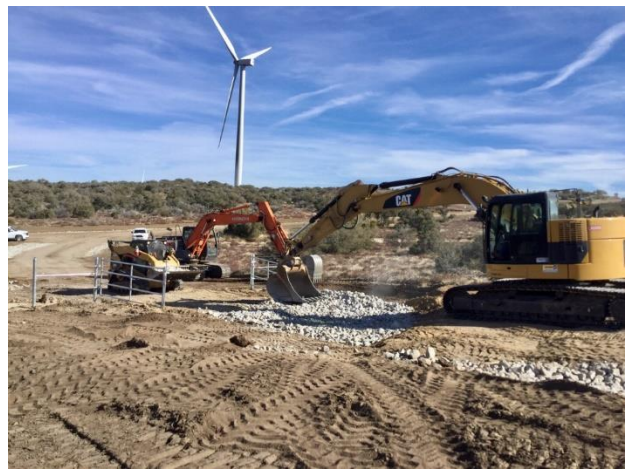
Photo 4: ECMs observed the construction of a low water crossing at the entrance of the B-line, within the approved limits of disturbance, in accordance with MM BIO-1a.
