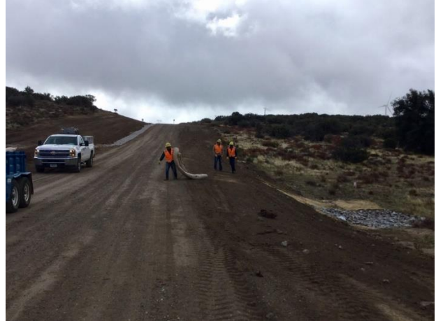
Photo 2: ECMs observed a construction crew removing old fiber roll debris found along McCain Valley Road. A biological monitor was present in accordance with MM BIO-1c.
