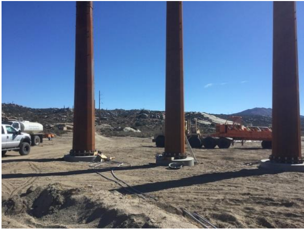
Photo 1: ECMs observed Mountain Power tightening sag points along the overhead collector line at Tower 66. The activity was spot checked by archaeological monitors per MM CUL-1d.
