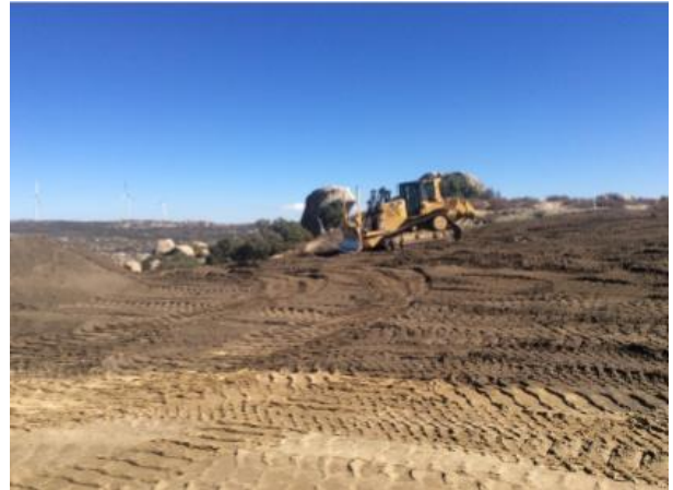
Photo 2: ECMs observed a bulldozer spreading topsoil along the G-line as part of site reclamation according to the Habitat Restoration Plan, MM BIO-1d.
