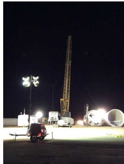
Photo 4: Light plants at turbine pad B-5 were positioned appropriately to minimize lighting in adjacent native habitats and the nighttime sky in accordance with MM BIO-7c, APM BIO-15, and MM VIS-3b.
