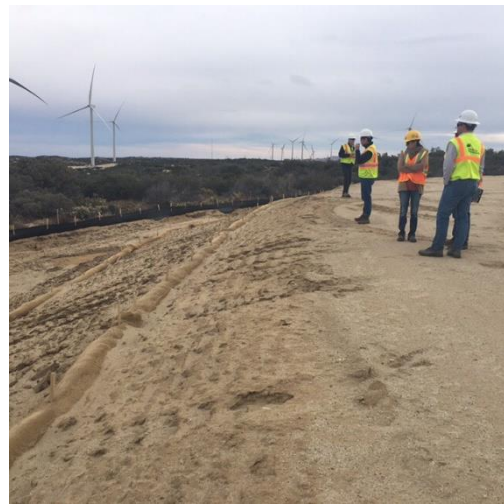
Photo 4: A SWRCB representative and representatives from Tule Wind LLC are observed inspecting slope grade and temporary straw wattle installation at turbine pad H-1 per the project specific SWPPP.
